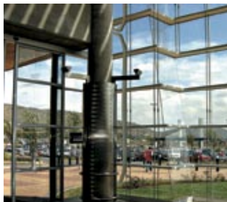
Clearwater Mall, Johannesburg Architect: Bentel Associates International Product: SmartGlass Solar E coated glass
