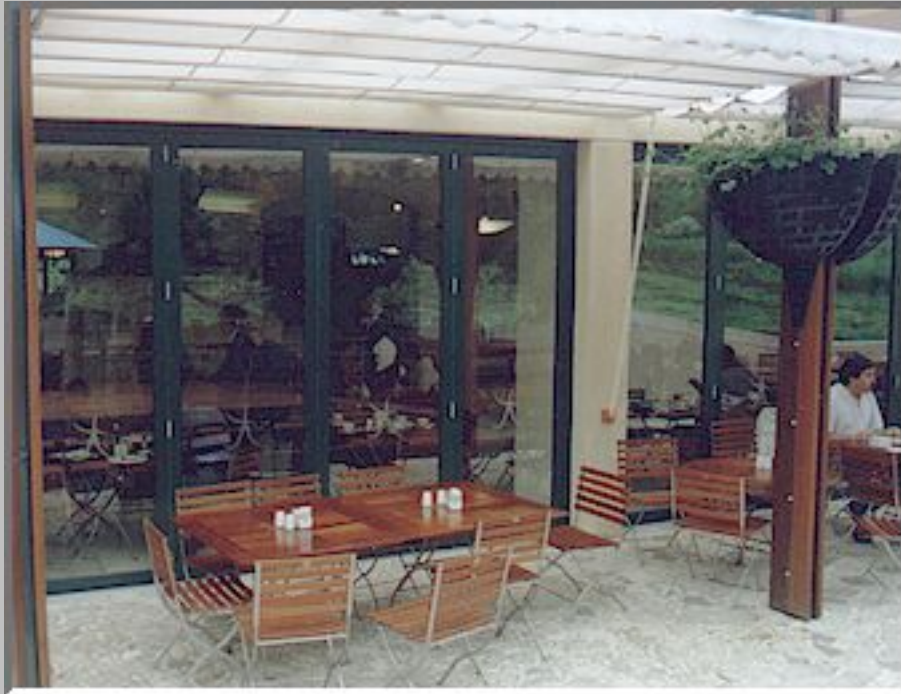
Kirstenbosch Restaurant - Kirstenbosch Cape Town Manufacture and installation of doors and windows.
