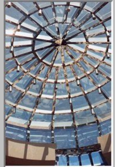
ALISSA SHOPPING CENTRE Al Khobar (Saudi Arabia) Design of aluminium and glass dome.
